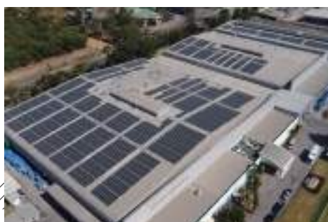
Solar Project Roongthavorn Plastic Co Ltd (RTP), Thailand
