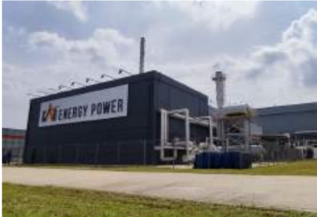
KAB Energy Power Sdn. Bhd.'s Safran Cogen Plant at Senawang, Seremban
